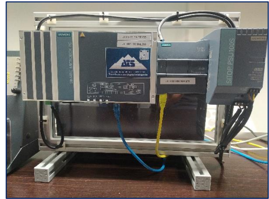
Figure 2: Industrial Edge Device y PLC
